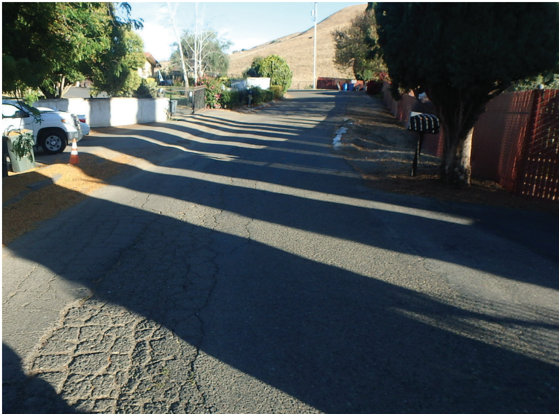
PHOTO 2: Area where water ponds. Also, note deteriorated roadway asphalt.
