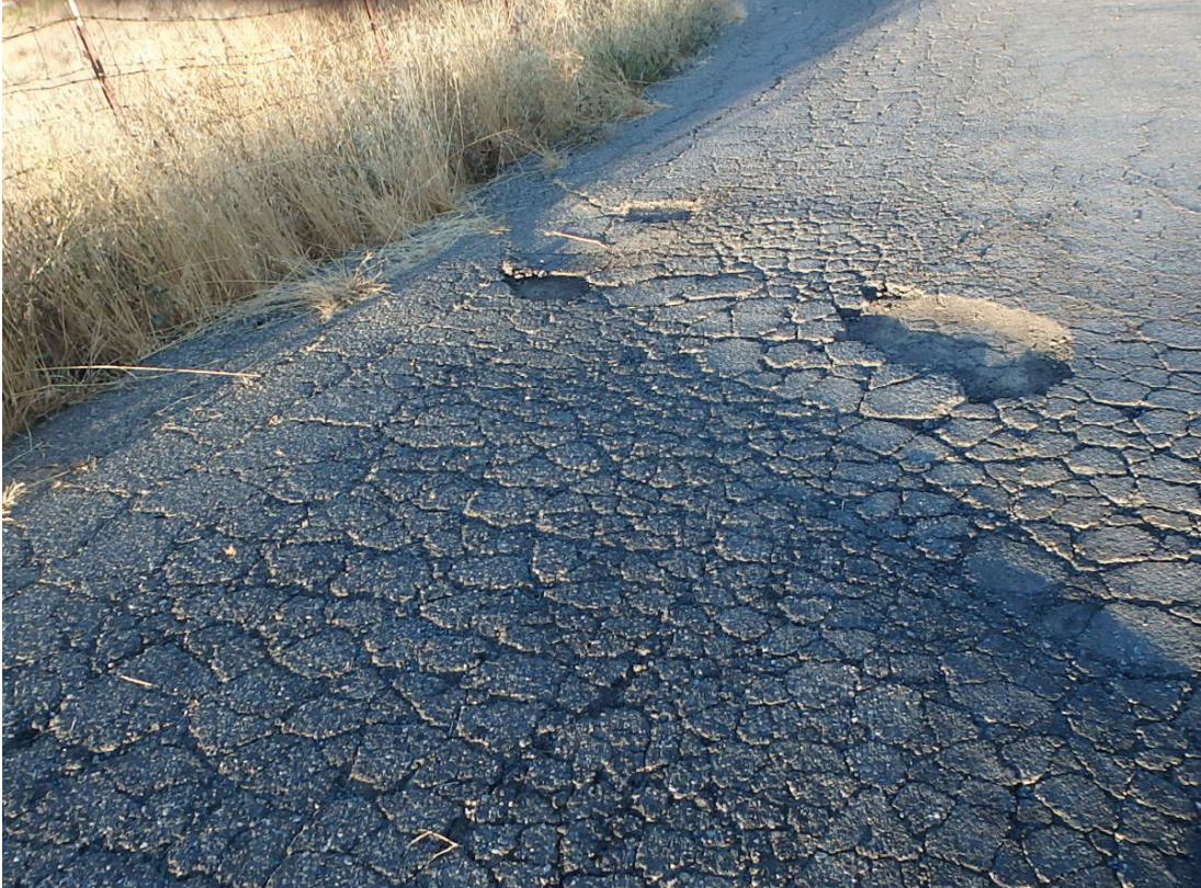
PHOTO 1: Typical roadway asphalt deterioration. Note “alligator” crack pattern and spalling of the upper asphalt overlay.
